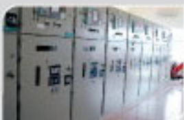
MV SWITCHGEAR CUBICLE
