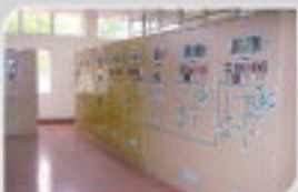
PROTECTION AND CONTROL PANEL FOR SUBSTATION
