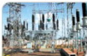
110KV KRONG BUK SUBSTATION
