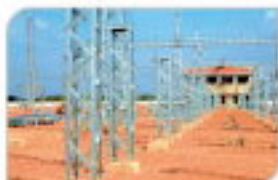
500KV TAN DINH SUBSTATION
